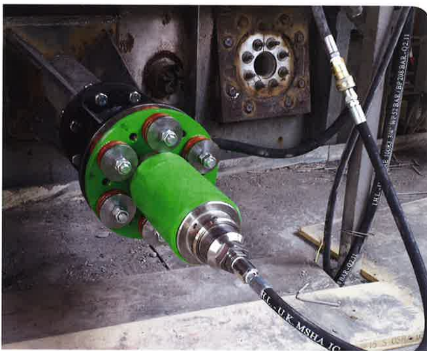
Turbo Flow installed at Giant Cement South Carolina.
